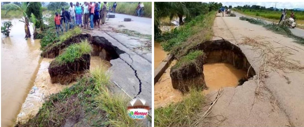
Figure 117: deterioration and destruction of the Santchou and Melon Road section due to heavy downpour on 21/08/2020.
