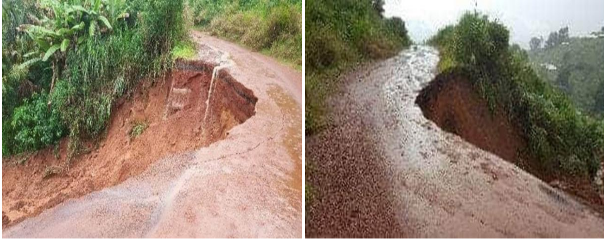
Figure 116: Landslide due to heavy rainfall in the Bui division on 17/07/2020
