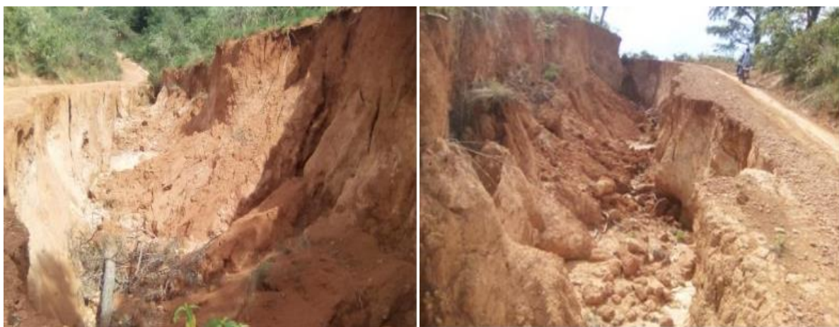
Figure 115: deterioration of the Lip-Mbokam Road section, Jakiri district, Bui division, North West region, in August 2020.
