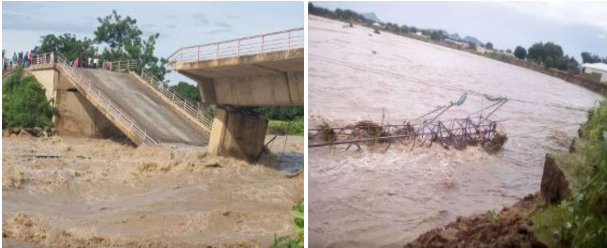
Figure 101: Collapse of the Palar bridge on the national road N°1 and destruction of the telecommunication infrastructure due to heavy rains on 31/08/2020
